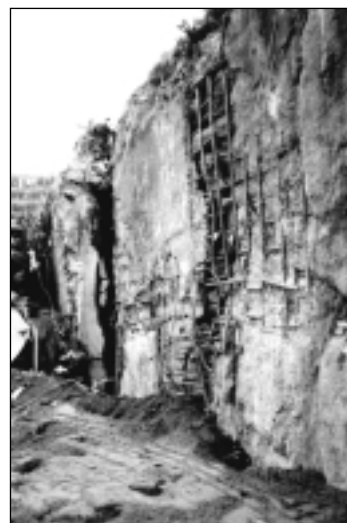
FIGURE 12 Damaged walls at Greenwich Street.
