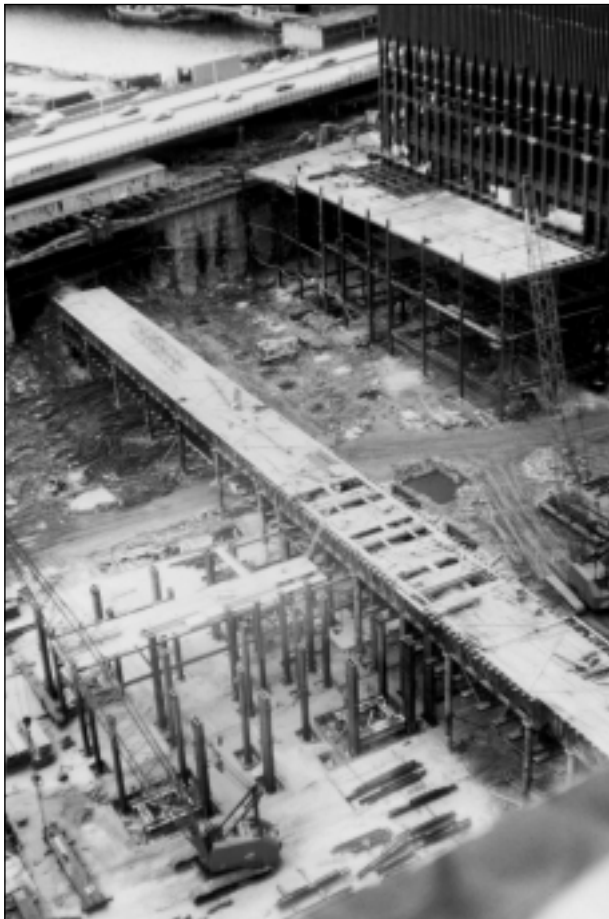
FIGURE 5 Original excavation, WTC 1 steel core started, PATH tubes temporarily supported while new station is constructed along Greenwich Street slurry wall.
