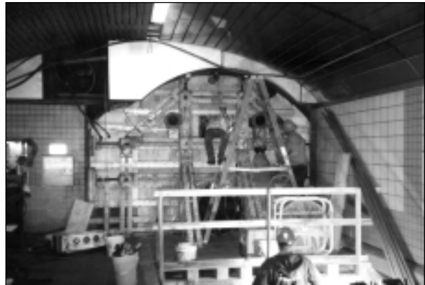
FIGURE 6 Current PATH tube plug at Exchange Place Station in Jersey City.
