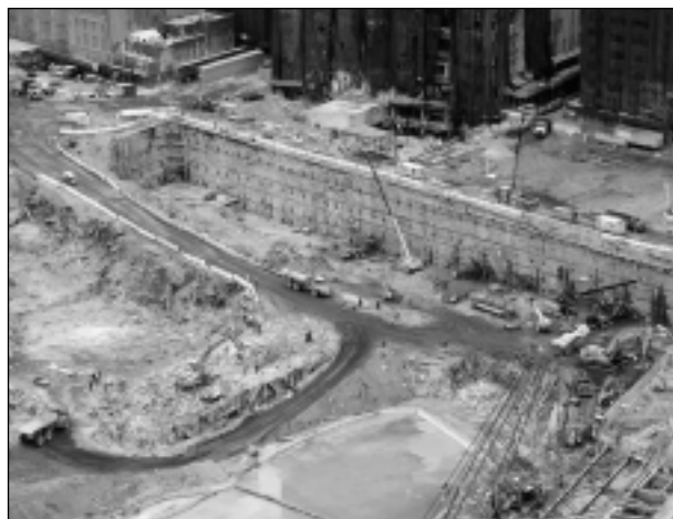
FIGURE 11 Progress along the Liberty Street slurry wall showing the installation of the fourth-tier anchors.
